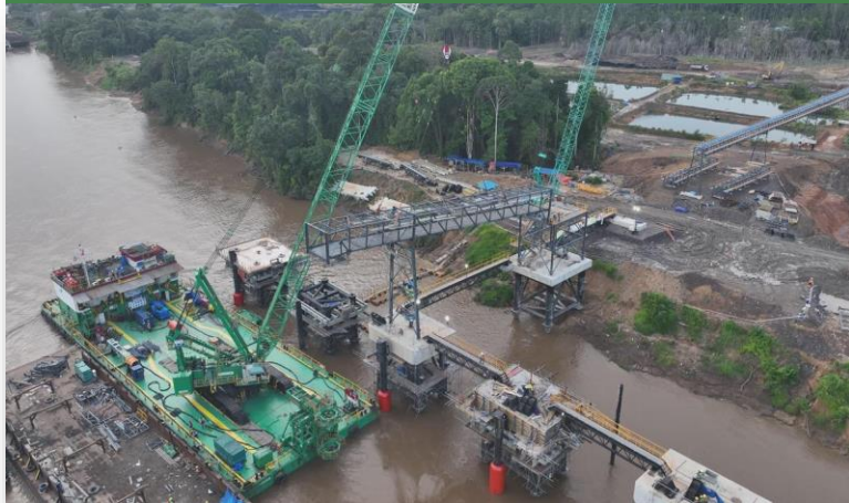
Second Barge Loading Conveyor
